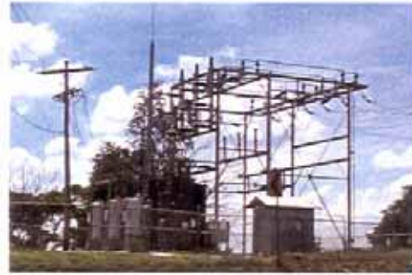
Truman Road and 7 Highway Substation
