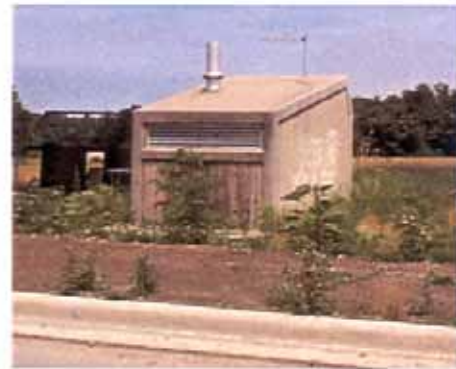
Little Blue Valley Sewer District meter station south of 39 th Street along the Little Blue Parkway
